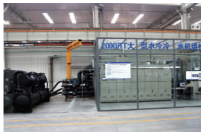
Water-cooled test lab up to 2000RT
